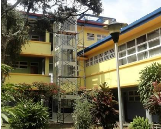
The newly installed elevator at the school
