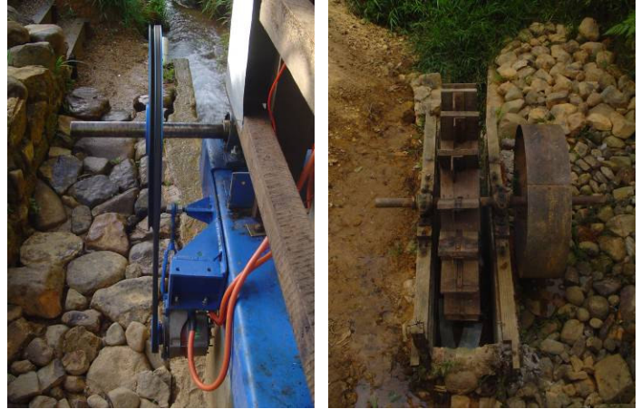
New and old components of the power generator
