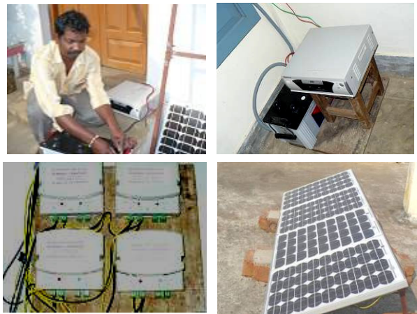
A technician installs the various components of a solar inverter power unit at a hostel in North India
