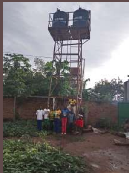
Chad: Construction of a bore hole and overhead tank for Academie St. Jean Paul II, Petit Seminaire, Moundou.
