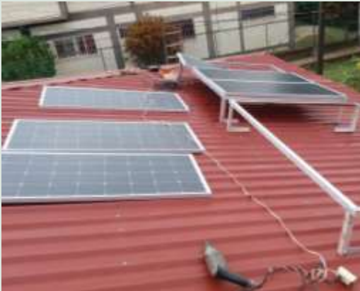
Honduras: Solar panels for the library and office at Puerto Lempira.
