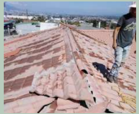
Costa Rica: A new roof for the formation house at Seminario San Vicente de Paúl.
