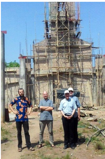
Superior General visits the Construction sight, Nov. 2018. From left: Fr. Paul Jakób, Fr. Jacob Hiler, Fr. Tomaž Mavrič, Fr. Stanislas Deszcz
