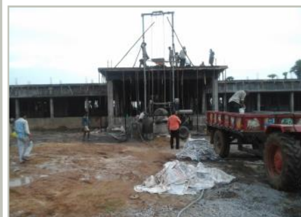
Construction of the ground floor of the school, 2017. Contractor Mr. G. Narayana Rao supervises the work.
