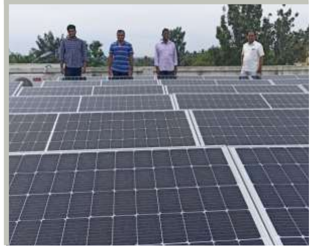
Fr. Anil Thomas CM, Fr. Jijo Joseph CM, Fr. Tibin Mathew CM, and Fr. Stephen Antony, CM of the South India Province on the roof of the provincial house with new solar panel bank installed.
