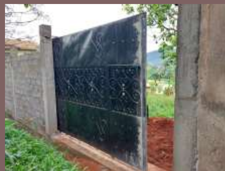
Cameroon: Construction of a gated wall for St. Vincent DePaul Yaoundé Major Seminary
