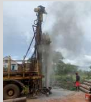
Sierra Leone: Water borehole for school complex
