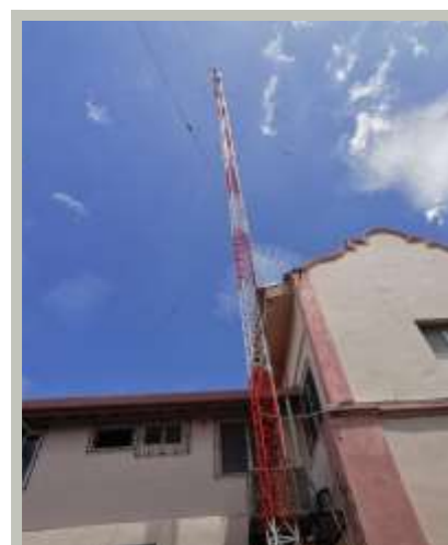
The new antenna reaches for the sky
