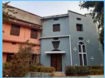
Renovation of Jyoti Nivas Minor Seminary at Baripadain the Mayurbhanj Seminary in India
