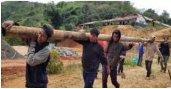
Construction of the parish community hall at De Paul Parish in Manipur, India
